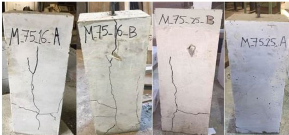
Fig. 5 Effect of increasing slab thickness on improving crack propagation in "M" specimens
